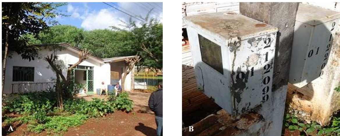
Figure 1. Consumer unit-CU (A) and residence entrance pattern (B)
