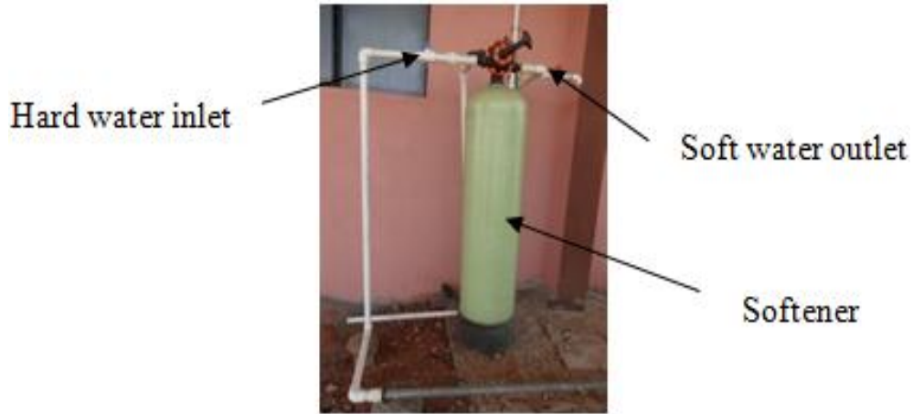
Fig. 1. Softener installed at dairy and food processing pilot plant
