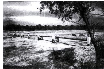
Fig. 6. Severe exposure of an oil pipeline through a dike in the northeast (1997 situation)
